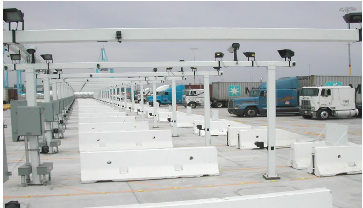
Figure 1: 24-lane Inbound Plaza Gate OCR Installation at Pier 400
